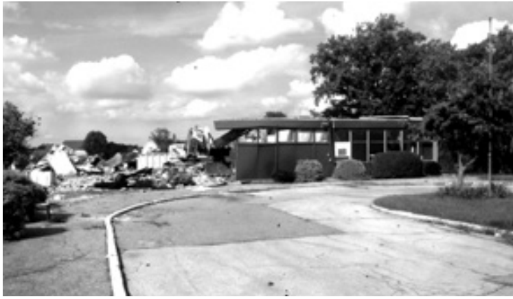
Demolition on the Old Seton Center began on September 9. The land on which the Old Seton Center previously stood will be returned to natural farmland.
