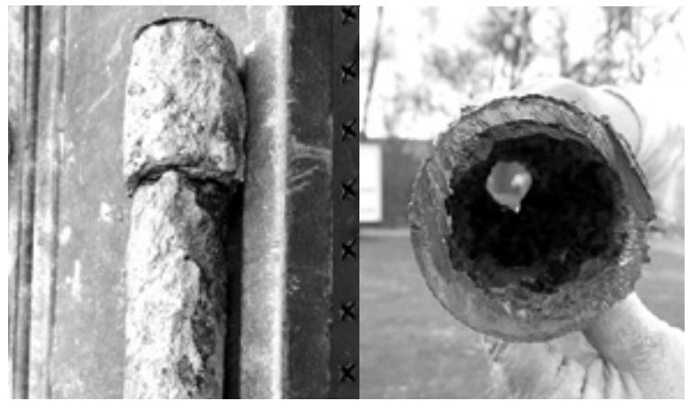
Crud and corrosion build-up in 70 year old pipes is the cause of Emmitsburg's brown water problem.
