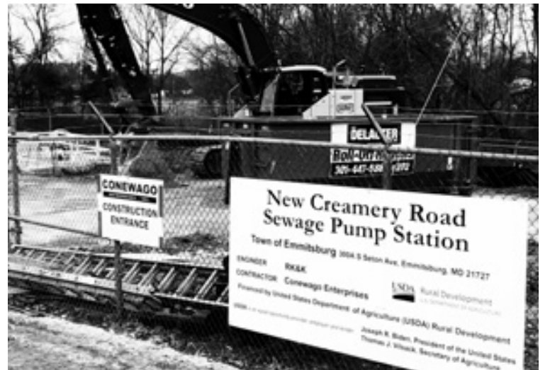
A good chunk of the Sewer Fund will be spent in the replacement of the Creamery Road sewage pumping station, the source of two recent sewage spills into Flat Run.
